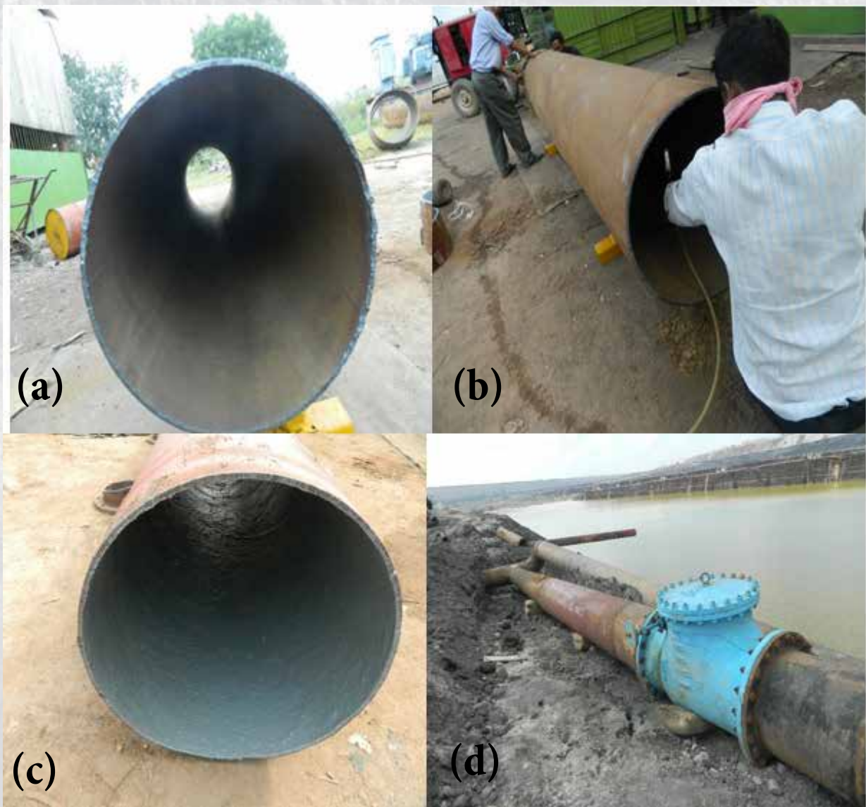
Fig. 1 Phase-I field trial: (a) Before coating (b) spray Coating (c) after coating (d) pipe being deployed in mainline
