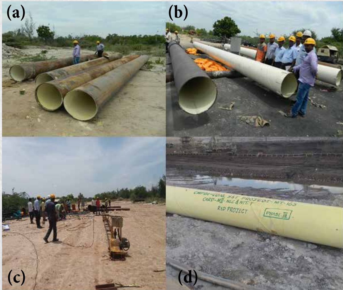
Fig. 4 Phase-III field Trail:(a) polyurea III coated pipes (Internal),(b) polyurea III coated pipes (Internal and external), (c) Movable Spray gun,(d) polyurea III coated pipes deployed in pipeline system
