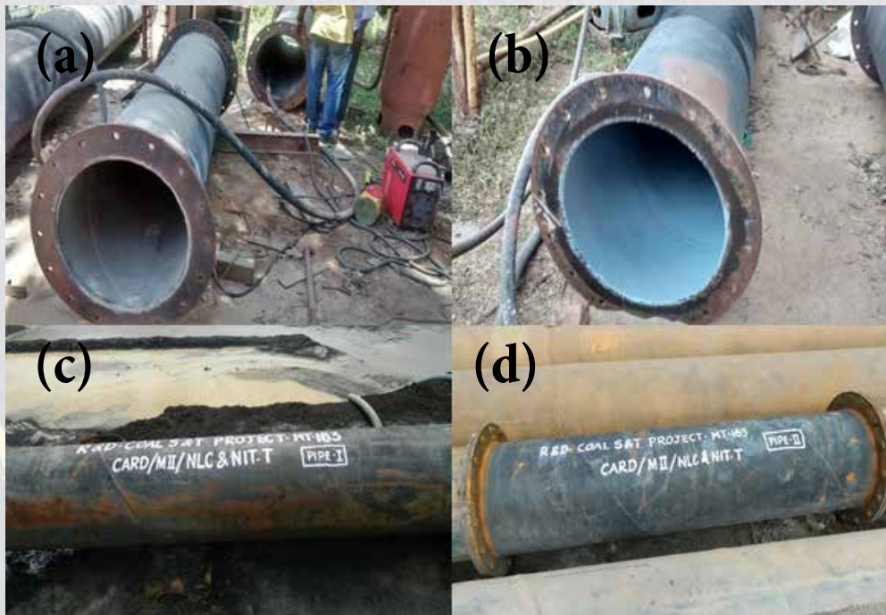
Fig. 2 Phase-II field trial :(a) Before coating (b) After Coating (c) Pipe-I being deployed in mainline (d) Pipe-II being deployed in mainline
